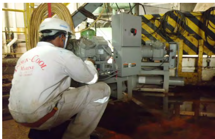
Provision Plant of Chillers Units
