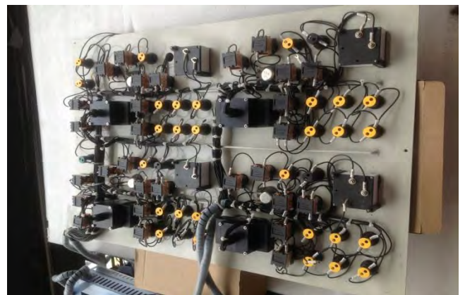
Electrical Control Switch(main board)
