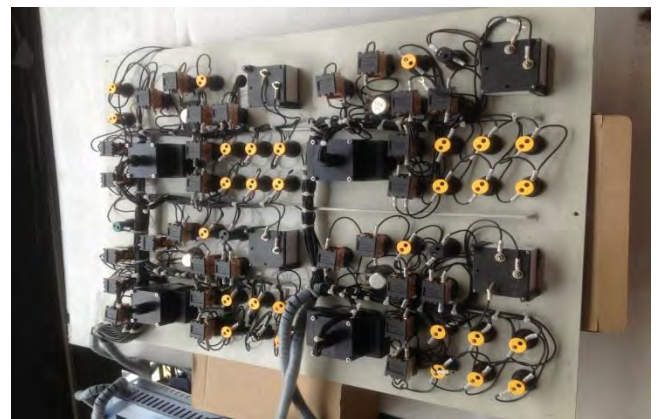
Electrical Control Switch(main board)
