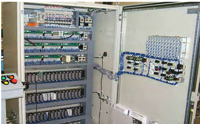
New Control Panel after Installation
