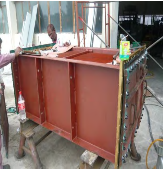
New Marine Engine of Aircooler fabrication
